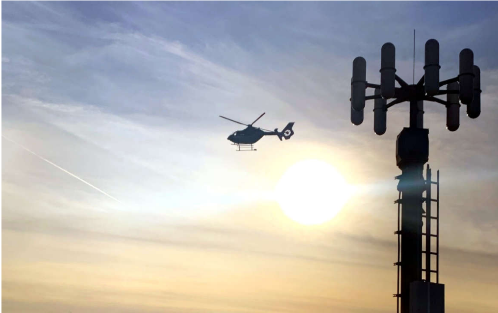
Field installation of the IZT R5509 direction finder in Wagenhausen.
