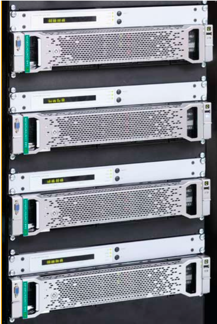
FIGURE 6: EXCEPTIONAL RELIABILITY AND FLEXIBILITY FOR DAB HEAD-ENDS
